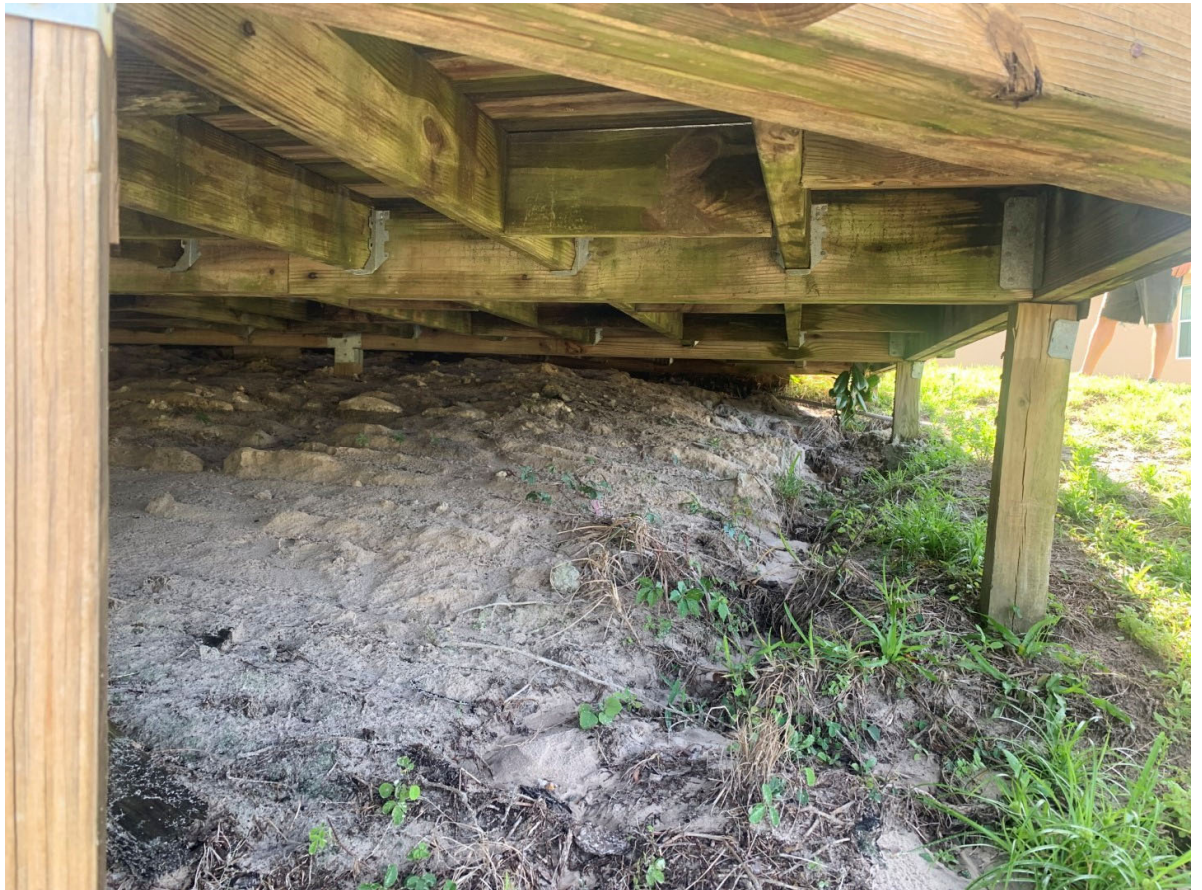
Channelized erosion present beneath deck and along side of property.
